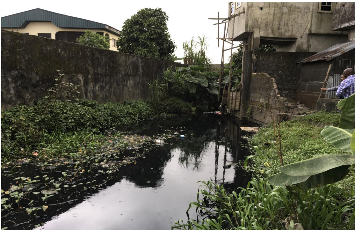
Figure 7: BLOCKED WATERWAY ON TORI CREEK, OFF JAKPA ROAD, EFFURUN
